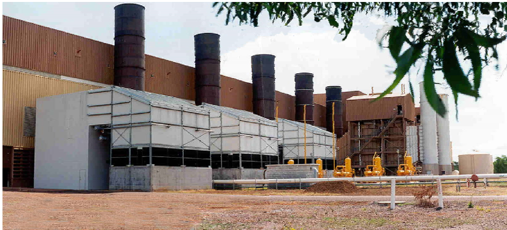
Figure 6: Wet Air Coolers at Channel Island Power Station
