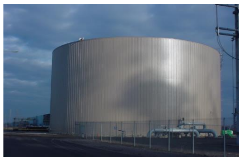
Photo 1 – 123,750 ton-hour (7.9 million gallon) CHW TES tank at Dominion’s Fairless Hills, PA plant (Photo credit: CB&I / McDermott)
