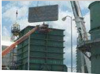
Exhaust Silencer Upgrades
