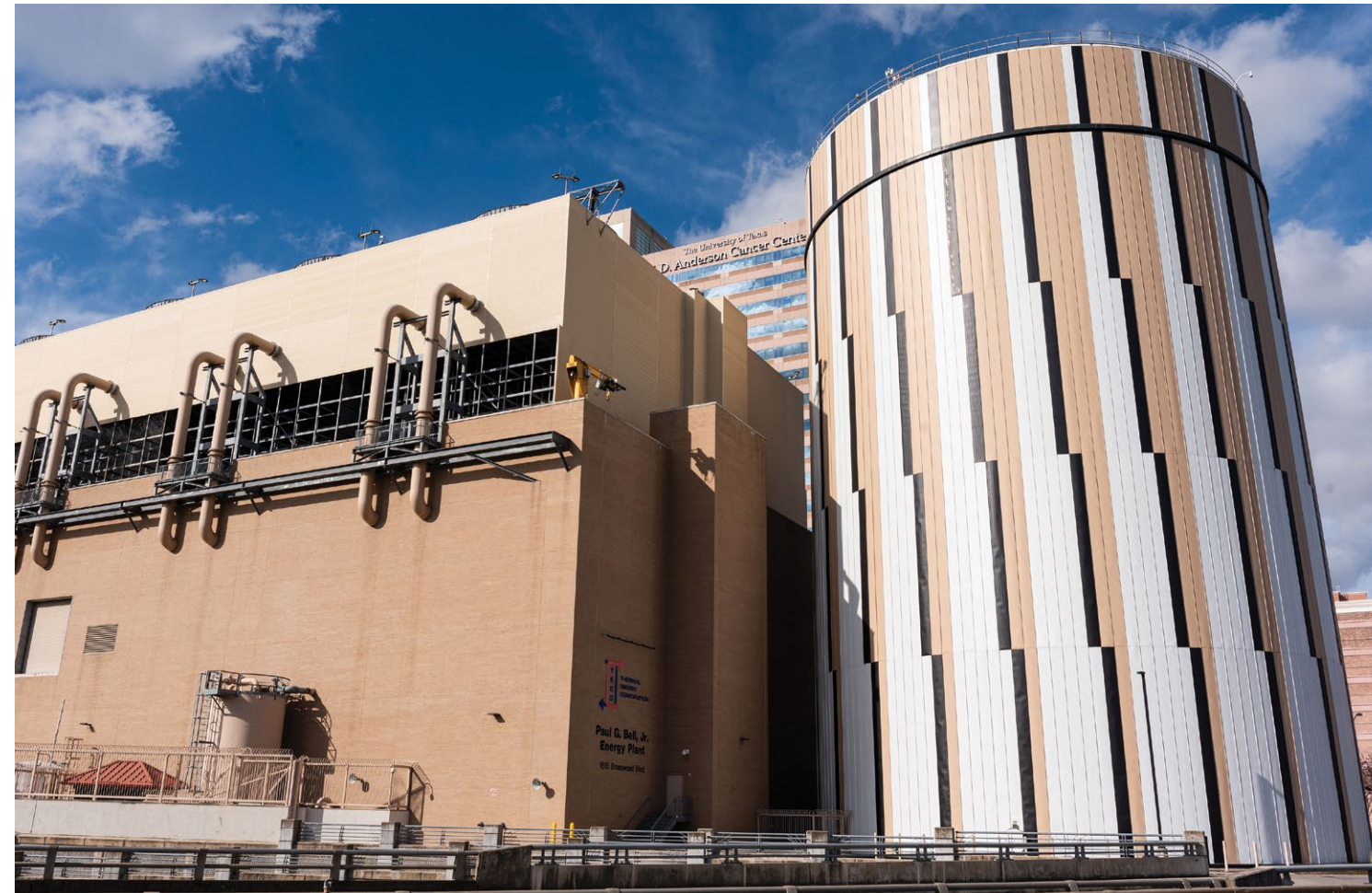
TECO's thermal energy storage and turbine inlet cooling are combined to enhance gas turbine performance.
